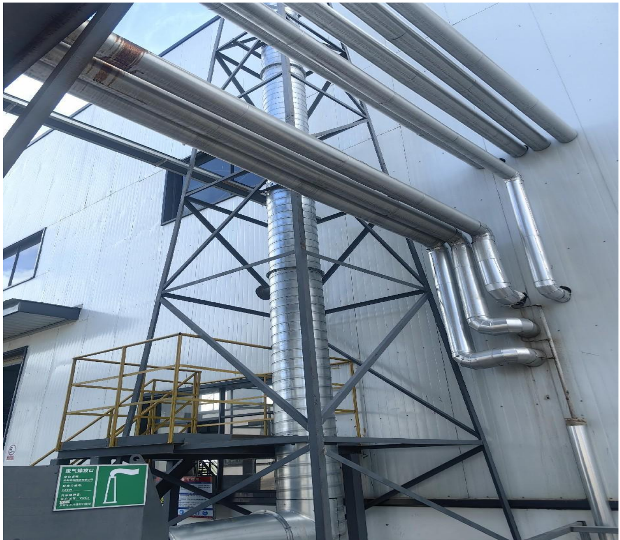
图4.1-1 废气排放口DA001
